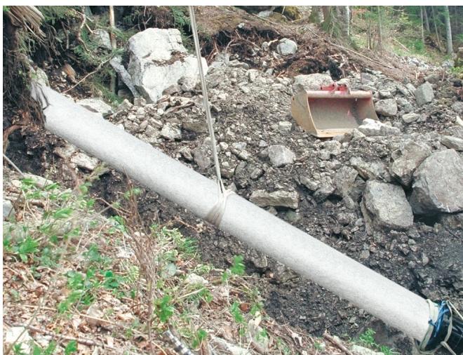
Protection against rockfall
